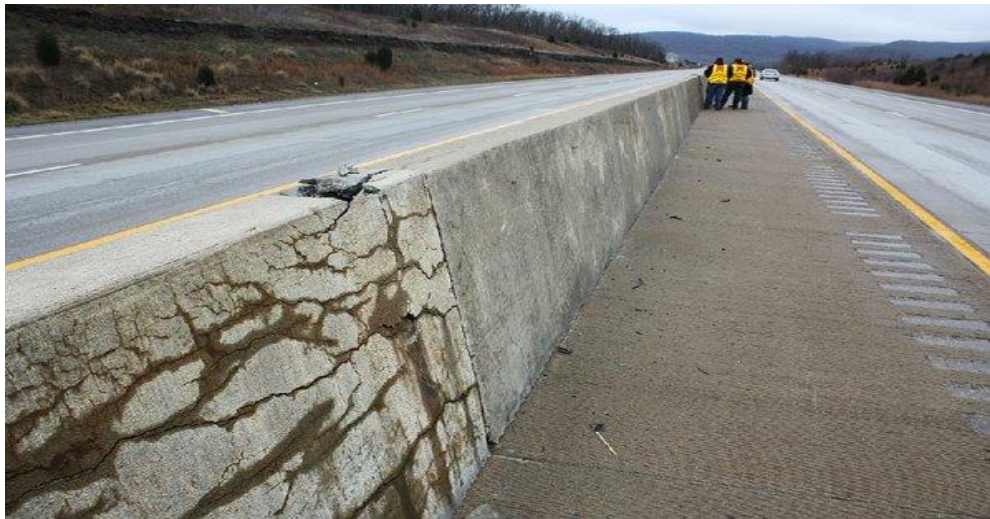
Figure 11: Cracked concrete median wall
